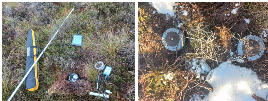
Figure 53: Field measurements (calibration) of water tables (left); installation of piezometers with lockable caps (right)
